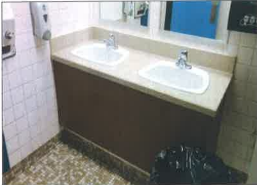
Upgrades are required in the washrooms to meet current barrier-free guidelines.
