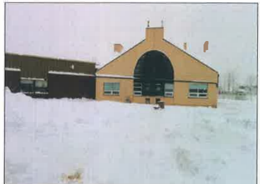
Pooling occurs on the site at the South moduls during spring thaw. Lighting levels should also be improved in this area.
