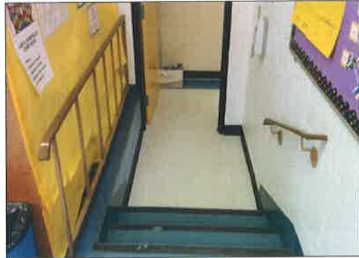
Accessibility to classroom 105 is an issue due to the space being the former stage.
