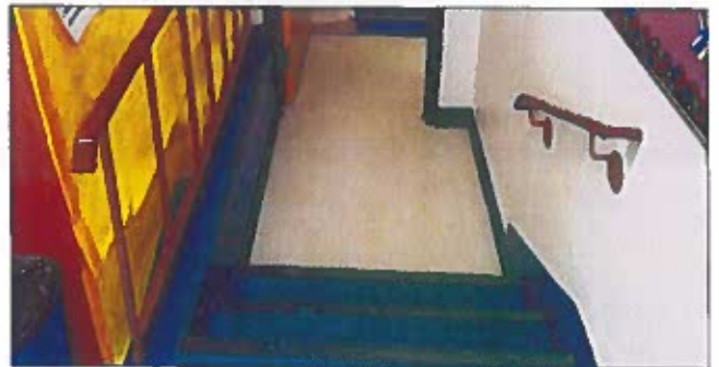
Accessibility to classroom 105 is an issue due to the space being the former stage.
