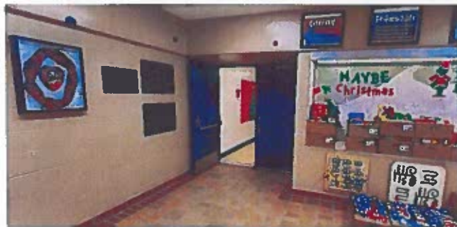
The single access point into the gymnasium causes congestion for students and community use.
