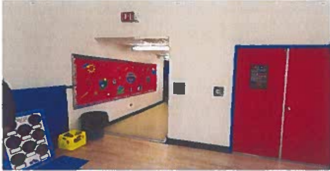
The single access point into the gymnasium causes congestion for students and community use.
