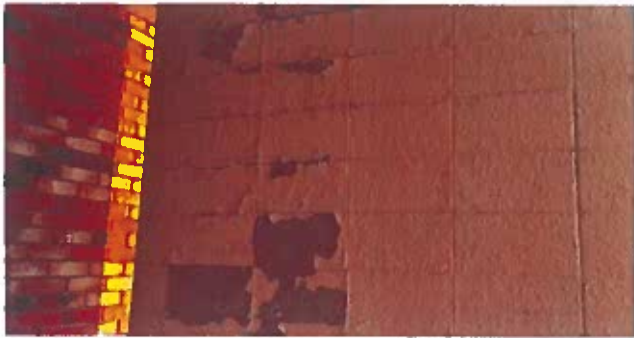
Spalling was noted on the exterior concrete block texture.
